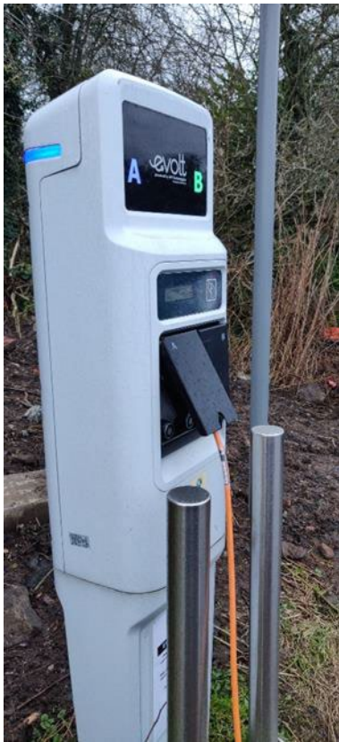
Figure 5.4 - EV charging point with protective bollards
