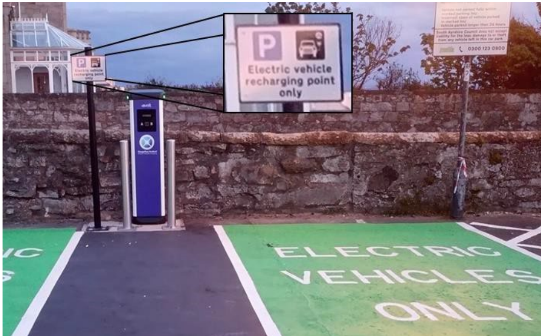
Figure 5.5 - EV charging bays with signage and markings
