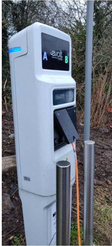
Figure 6: EV charging point with protective bollards
