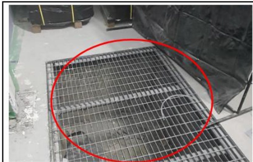
Photo No. 2: The cubicles of the E&I Form 4b type 6 low voltage switchboard are ready to be joined together and mounted over the steel grating.
