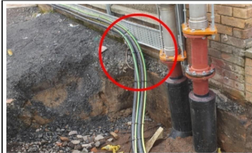
Photo No. 1: The parallel feeder cables (i.e., 2No x 4Core x 150mm SWA cable complete with 150mm 2 supplementary earth(s) have been installed.
