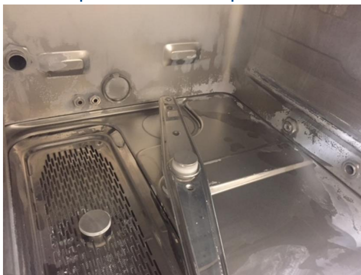
Image 3.1: An example of lime scale build-up within a washer disinfectator
