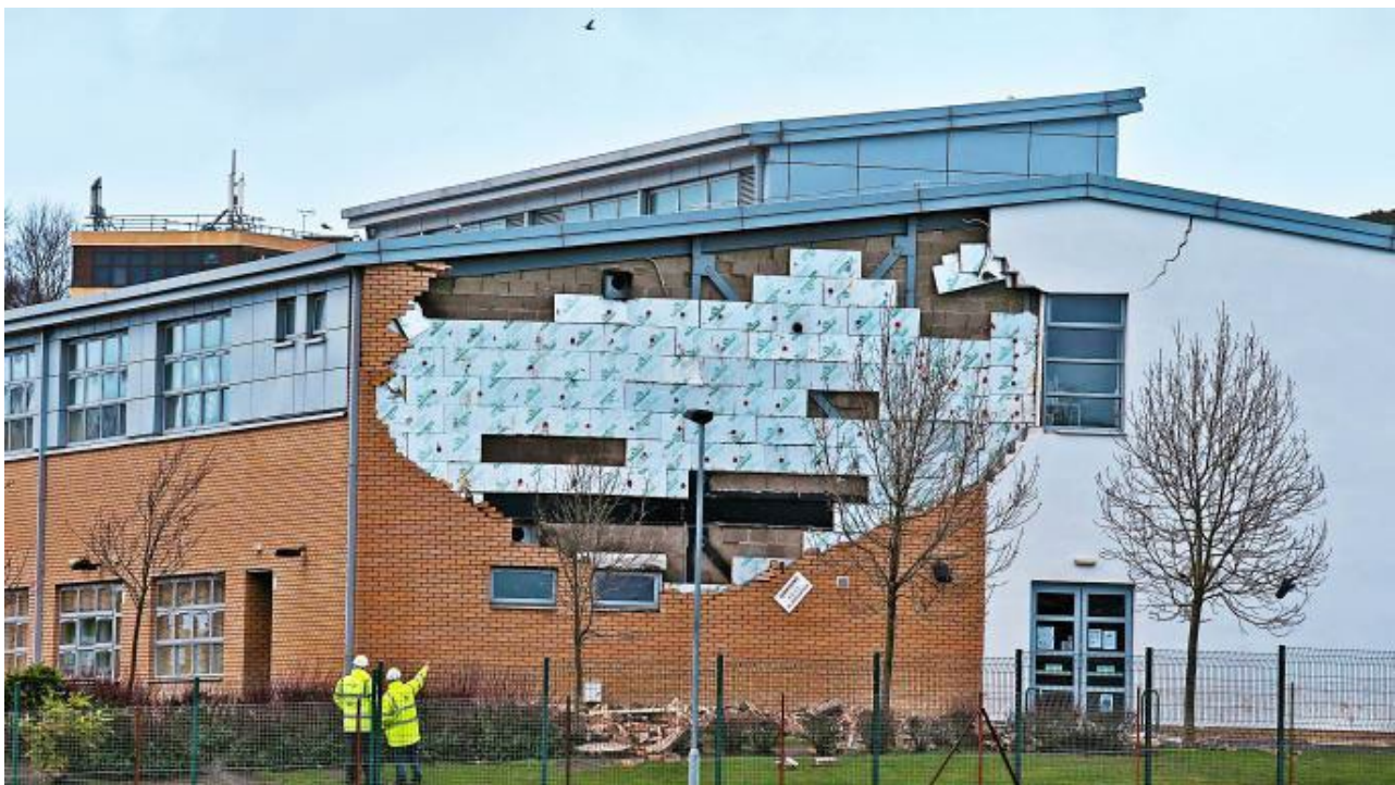
Figure 2: Oxgangs Primary School collapsed wall following high winds January 2016
