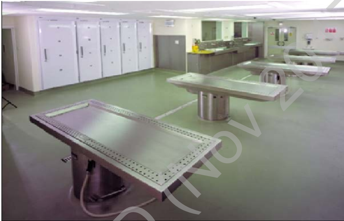
Post-mortem room showing down-draught ventilated post-mortem tables and pull through fridges
