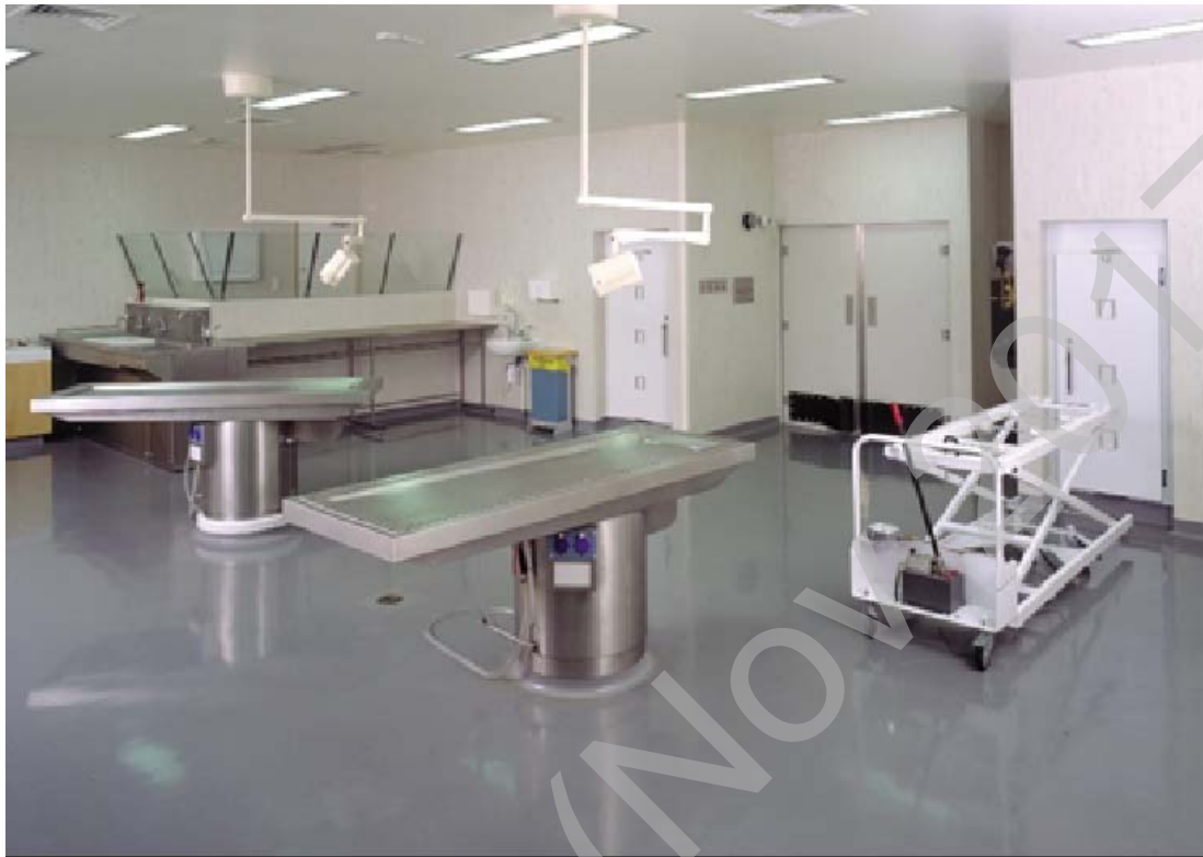
Post-mortem room showing adjustable-height mortuary trolley
