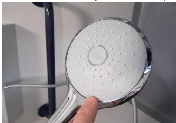
Check shower head for any residue or build up of lime scale.
