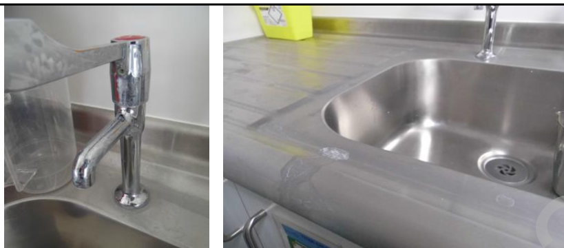
Build up in sink drain.
