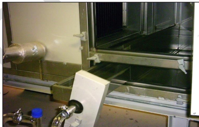
Figure 7 Removable AHU drainage tray
