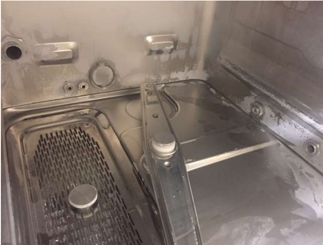
Figure 2: An example of lime scale build up within a washer disinfector
