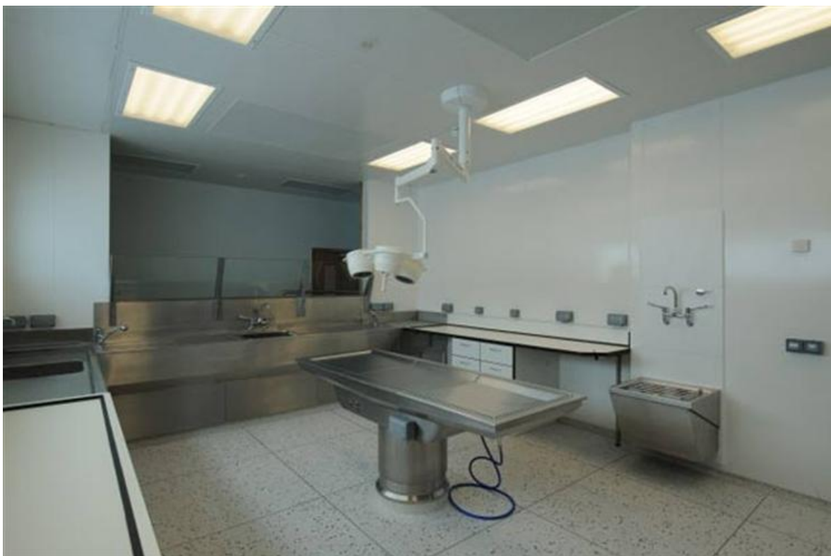
Figure 5-13: Open plan observation area, in 'high risk' PM room, Royal Victoria, Belfast
