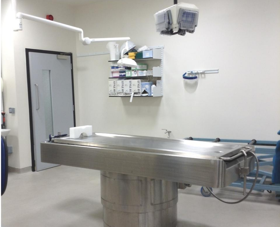
Figure 5-10: Single, segregated PM table in 'high risk' room, QEUH, Glasgow
