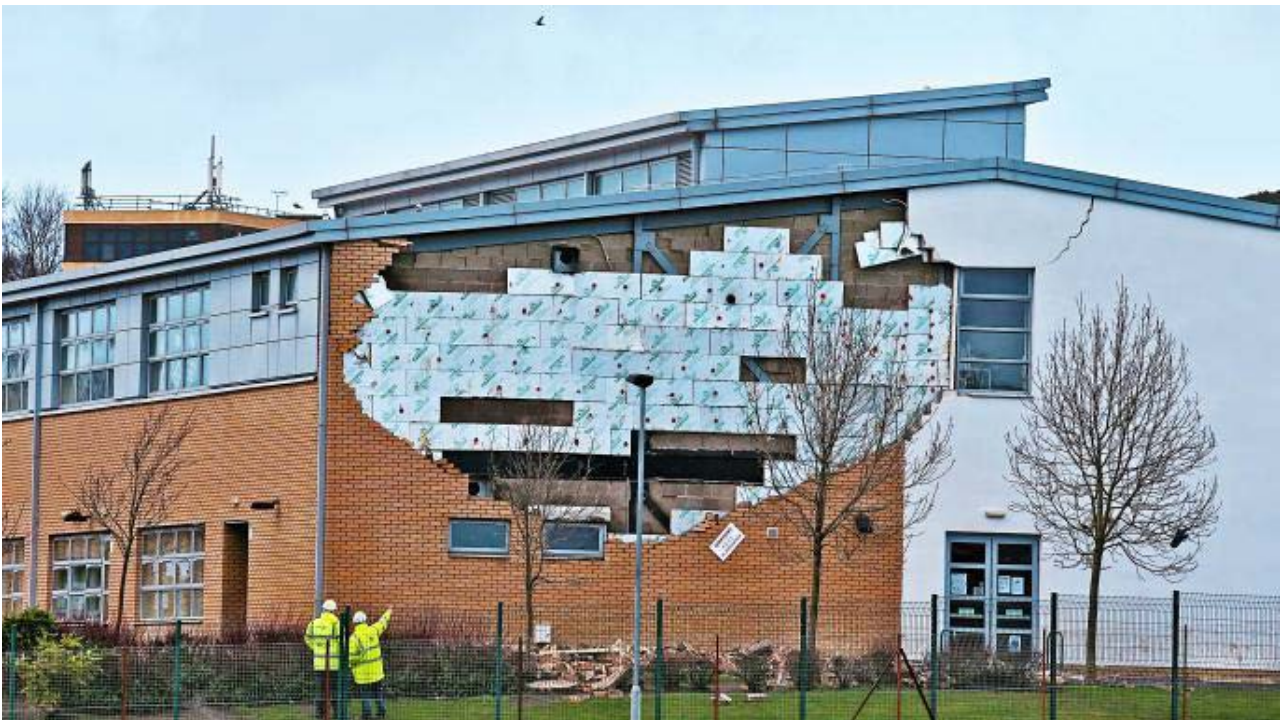
Fig 2 A wall collapsed at Oxfangs Primary School during high winds in January 2016
